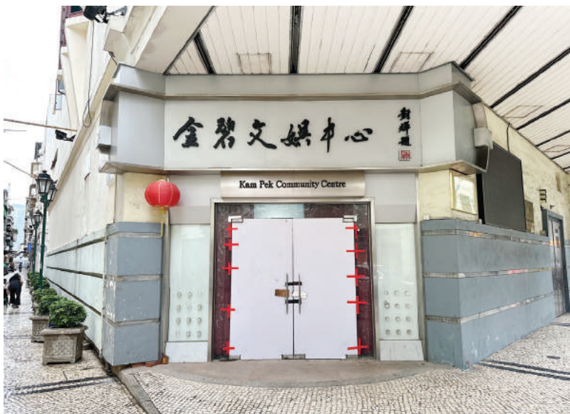
This photo taken yesterday shows the under-renovation Kam Pek Community Centre on Avenida de Almeida Ribeiro.
