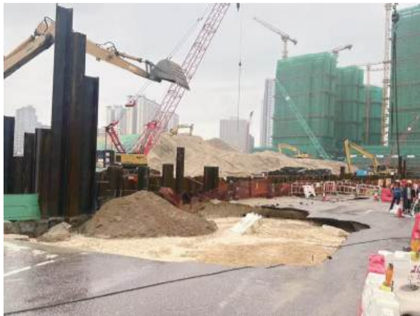
This handout photo released by the Public Works Bureau (DSOP) yesterday shows the sinkhole at a location where Rotunda de Hou Kong meets Avenida Doutor Ma Man Kei in Zone A.
