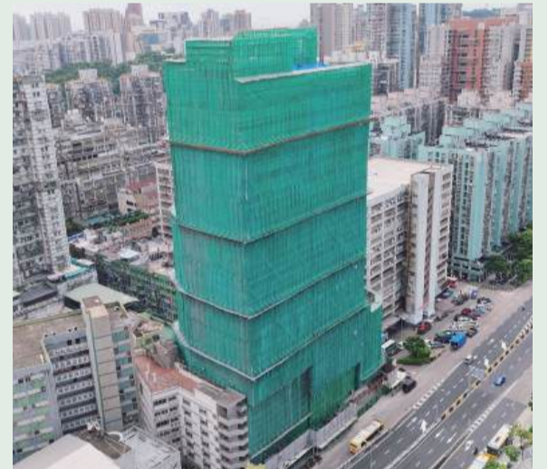
This file photo taken by the Public Works Bureau (DSOP) in June shows the redevelopment project of the Housing Bureau headquarters in Patane.
