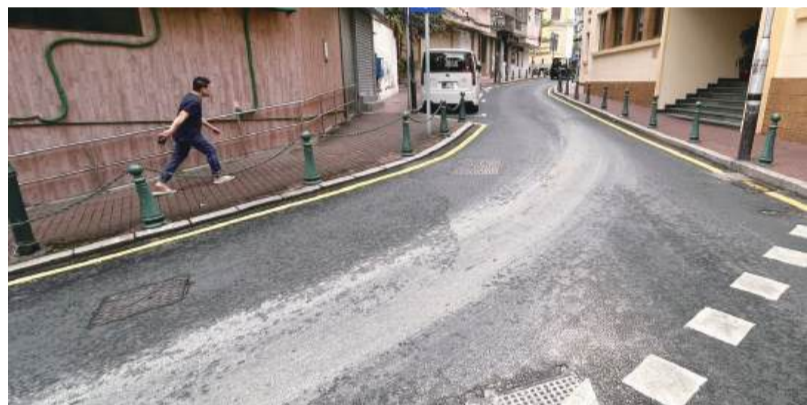
This handout photo provided by the Municipal Affairs Bureau (IAM) yesterday shows cement slurry left on Rua da Imprensa Nacional (官印局街).
