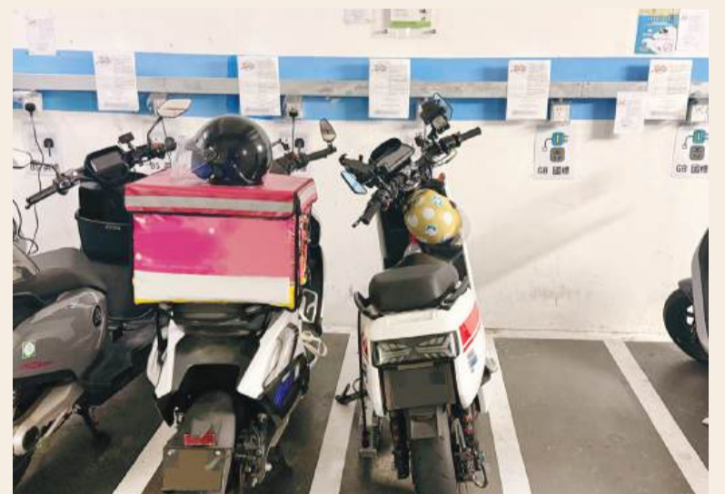
This undated handout photo provided by the Environmental Protection Bureau (DSPA) last Tuesday shows the charging station for e-motorbikes in a public carpark.
