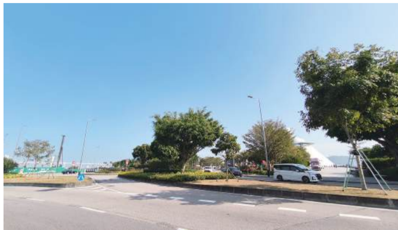
Vehicles drive along Avenida Dr. Sun Yat-Sen on the Nape waterfront near the Macau Science Centre (MSC) earlier this month where construction of a sea-crossing flyover linking with Zone A (left) started late last year. — Photo: Tony Wong
